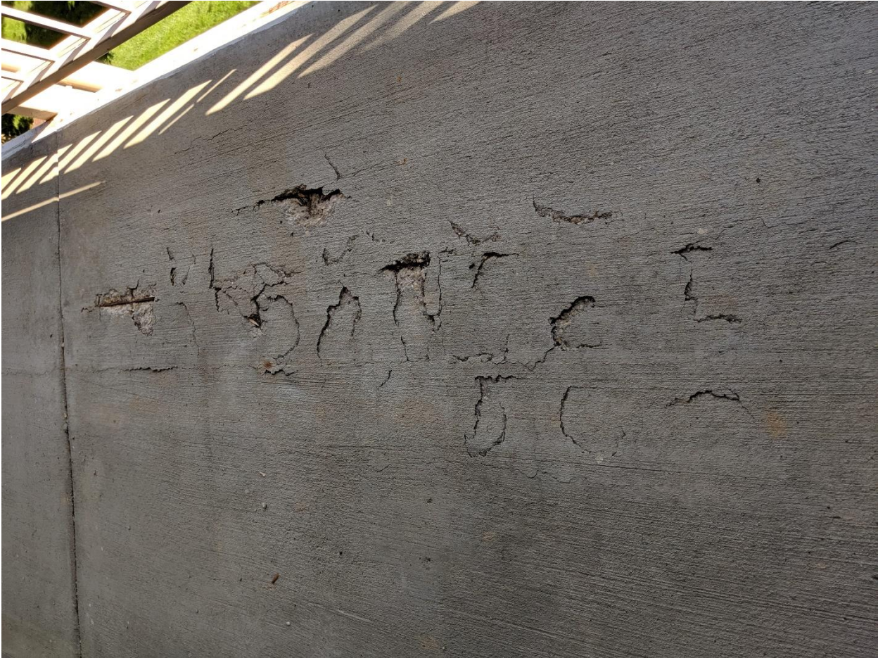
B15-3F Balcony concrete damage
